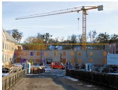
Fig. 37. Courtyard elevation of the south wing, after hacking off plaster and dismantling roof rafter framing, before building the tower. Chronological stratification of walls: A – walls of the building from phase IV altered in stage I of phase VI; B – walls from stage I of phase VI altered in stage I of phase VII; C – walls from stage I of phase VII. Photo by L. Wawrykiewicz, 2010
