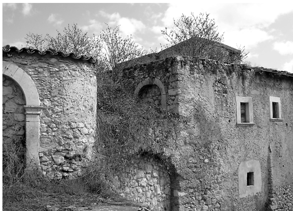
Fig. 1. The state of conservation of the existing masonry buildings
