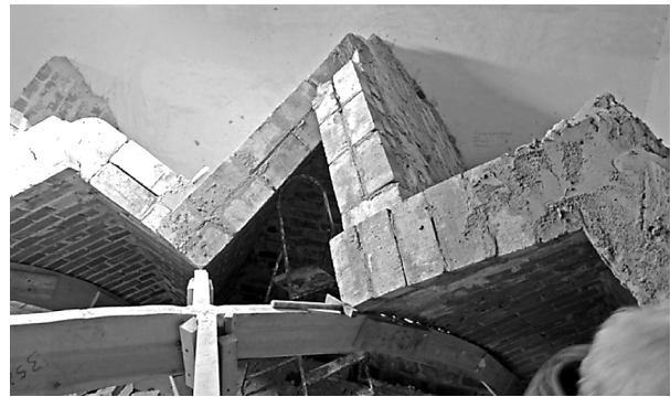
Fig. 13. Also in the higher portions the continuity over the whole squinch can easily be maintained. Over the transversal cap, the courses are seamed (D. Wendland)
