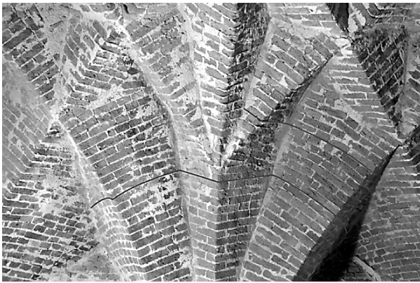
Fig. 8. The exposed masonry texture of the analyzed vaults shows the continuity of the courses over large portions, across the discontinuities of the vault surfaces (cf. also Figure 3). This is not conform with modern masonry rules and contradicts the current descriptions models, but in the experiments turned out to be very practical (D. Wendland)
