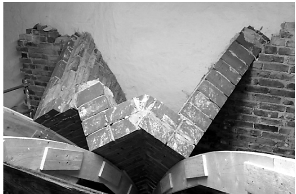
Fig. 11, 12. Details of the experimental reconstruction. The vault masonry is executed without formwork on single centering arches supporting the groins. The thickness of the shell is according to the archaeological evidence. The peculiar masonry texture with the continuity of the courses over the inward folds, as observed on the original vault, turned out to be practical (D. Wendland)
