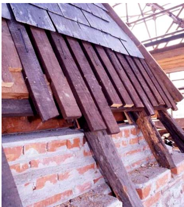
Figs. 18–19. Connection between rafters and girds via steel pins to get the continuity of roof pitch
