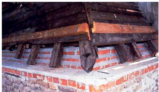
Figs. 16–17. Area of the masonry wall supporting the timber carpentry before (Fig. 16) and after (Fig. 17) the intervention (1986)
