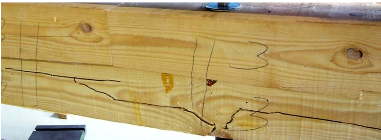
Fig. 16. Specimen 03 – fracture next to a knot on the bottom surface
